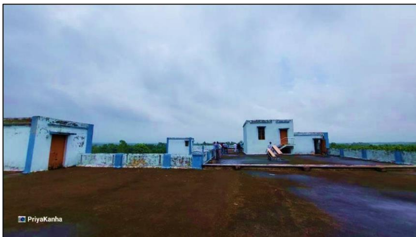
Plate 21: The vast terrace of college has high potential for Solar panel installation (Source: Dr. Priyanka Halder Mallick)
