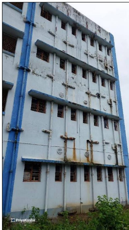
Plate 17: Sanitary pipes are damaged (Source: Dr. Priyanka Halder Mallick)
