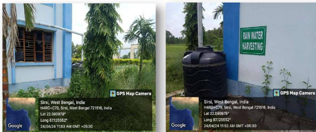
Plate 2: Rainwater Harvesting System in the College Campus (Source: College authority)
